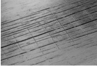
Weathered wood structure *
